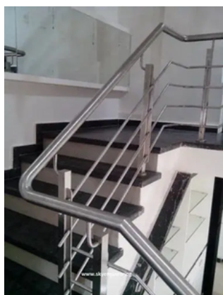
Stainless Steel Ramp Railing
